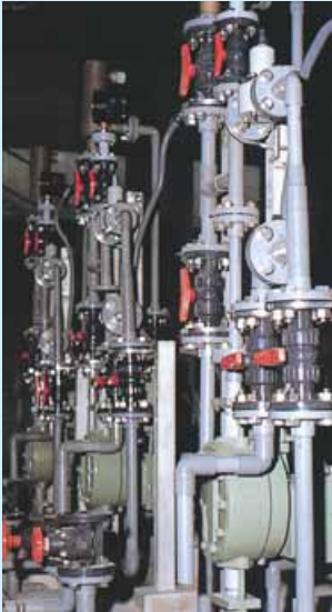
Chemical Treatment Piping for water purification system
