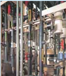
High purity EsloClean piping
