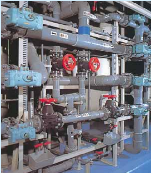
Water treatment piping for electronics factory
